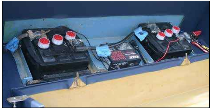
Older style dual wet cell 6V battery installation.
